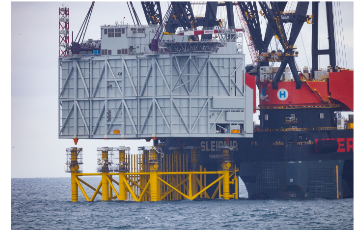
August 2024 installation of an HVDC offshore converter platform at RWE's Sofia Wind Farm, off the coast of the United Kingdom. (Image credit: RWE)
