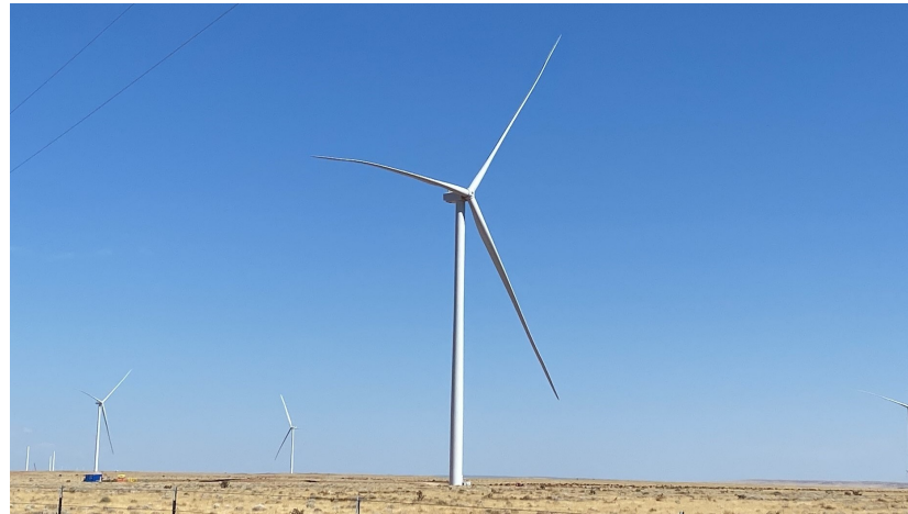
First of 674 3.6MW-154m workhorse turbines that will provide 2.4 GW+ of power installed at Pattern Energy's SunZia Wind Project in New Mexico, expected to be the largest wind project in the Western Hemisphere.
